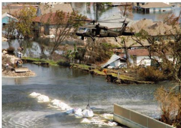
Through the breach. Engineers say the 142-meter gap in the 17th Street levee was caused by a damaged foundation. It took 5 days to close.
